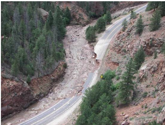
Figure 2.29 – West Creek Highway 67 Shoulder Damage Photo courtesy of CDOT
