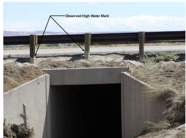
Figure 3.9 – Bosley Wash – I-70 High-water mark on guard rail, upstream end of culvert
