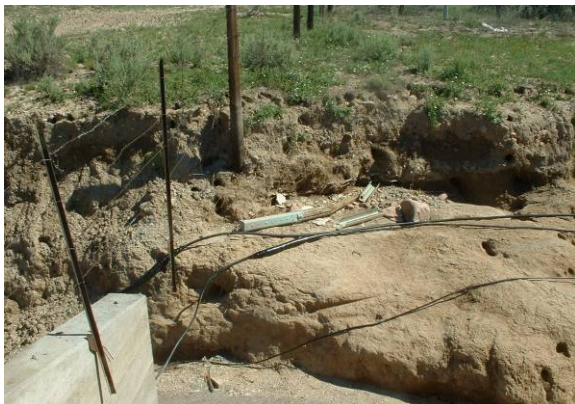
Figure 1.26 – Brush Hollow Creek Highway 50 Bridge Utility Damage, Westbound Bridge
