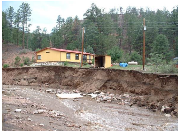
Figure 2.36 – West Creek – Private Residence Isolated by Bank Erosion
