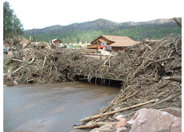
Figure 2.22 – West Creek – Bailey Residence at 15590 West Creek Road. Box culvert is 16' x 6' in size. Water surface was 6 to 8-inches above first floor level in house.
