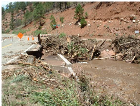
Figure 2.34 – West Creek - Highway 67 Damage
