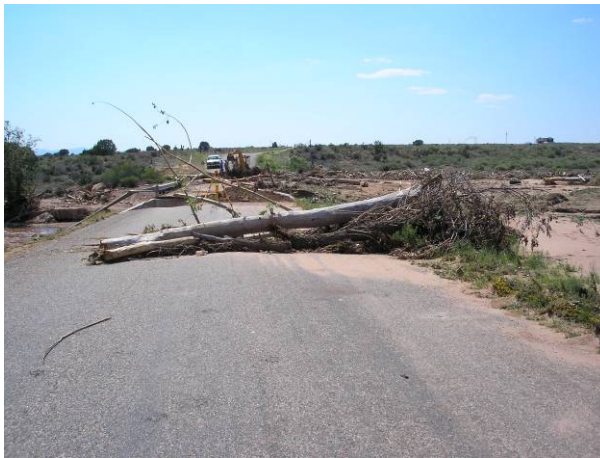
Figure 1.33 – County Road 123 at Eightmile Creek Bridge Overtopping, Crest of Road at Bridge
