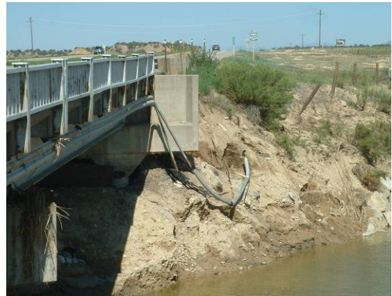
Figure 1.25 -- Brush Hollow Creek Highway 50 Bridge Looking Upstream – Utility Damage
