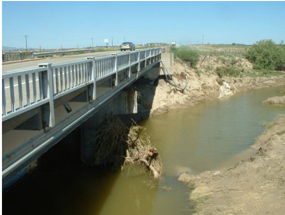
Figure 1.24 – Brush Hollow Creek Highway 50 Bridge Looking Upstream Note: high-water came up to low steel elevation resulting in minor overtopping of westbound lanes.
