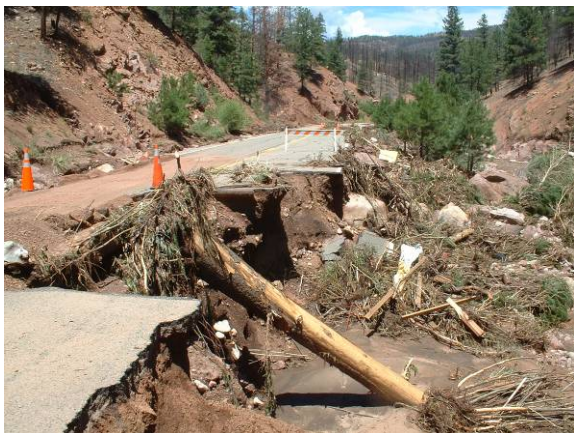
Figure 2.33 – West Creek - Highway 67 Damage
