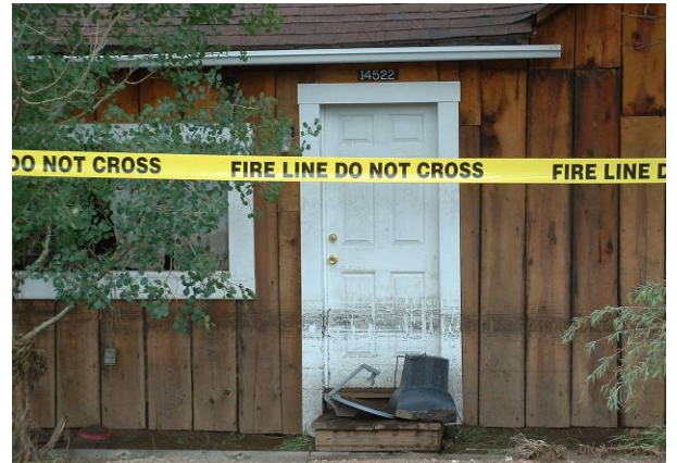
Figure 2.24 – West Creek – High-water Mark on Residence Upstream of Culvert Crossing at Abbey Avenue.
