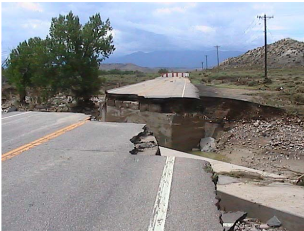
Figure 1.22 – Brush Hollow Creek Highway 115 Culvert Overtopping
