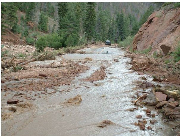
Figure 2.37 – West Creek – Highway 67 Road Overtopping
