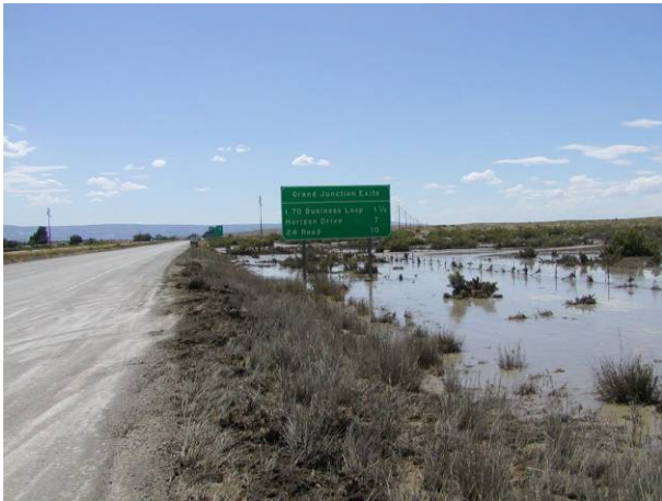
Figure 3.10 – Bosley Wash – I-70 Ponding along northern edge of roadway
