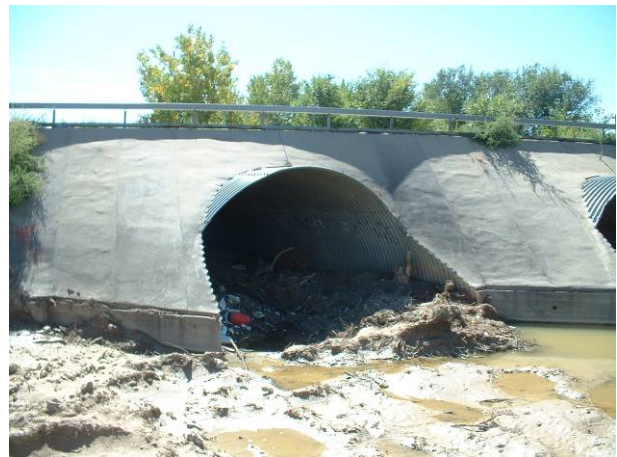
Figure 4.17 – 18 th Street Bridge – Middle Culvert at Wild Horse Creek – Note sediment and trash.
