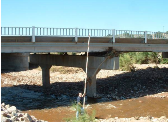
Figure 1.28 – Highway 50 Bridge – Eightmile Creek Looking Downstream Note debris on top of pier cap.
