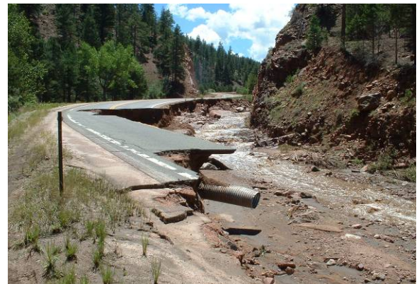
Figure 2.32 – West Creek - Highway 67 Damage
