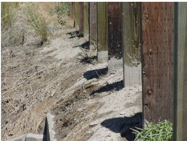
Figure 3.8 – Bosley Wash – I-70 Culvert mud level on guard rail
