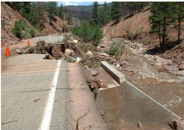
Figure 2.31 – West Creek - Highway 67 Box Culvert Damage
