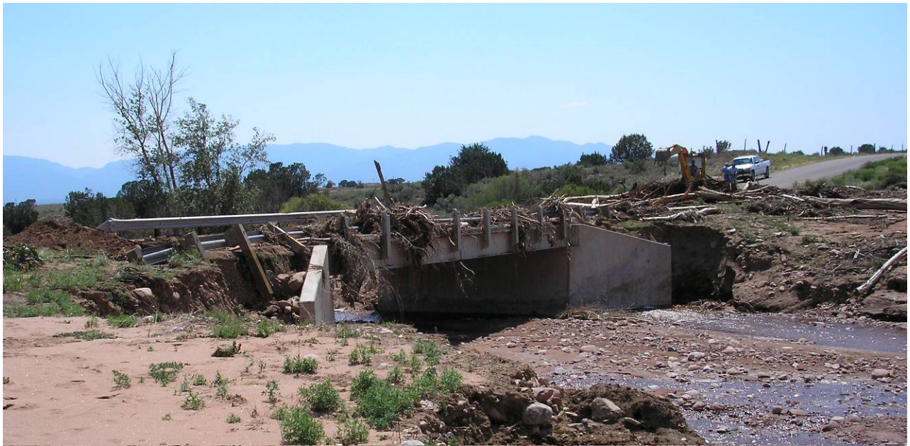
Figure 1.30 – County Road 123 at Eightmile Creek Bridge, Overtopping Upstream Face.
