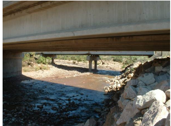
Figure 1.29 – Highway 50 Bridge – Eightmile Creek Looking Upstream Note minor erosion along toe of slope.
