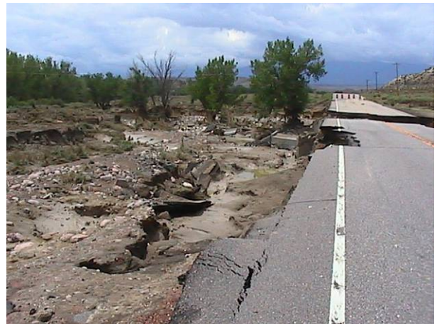
Figure 1.23 – Brush Hollow Creek Highway 115 Road Damage
