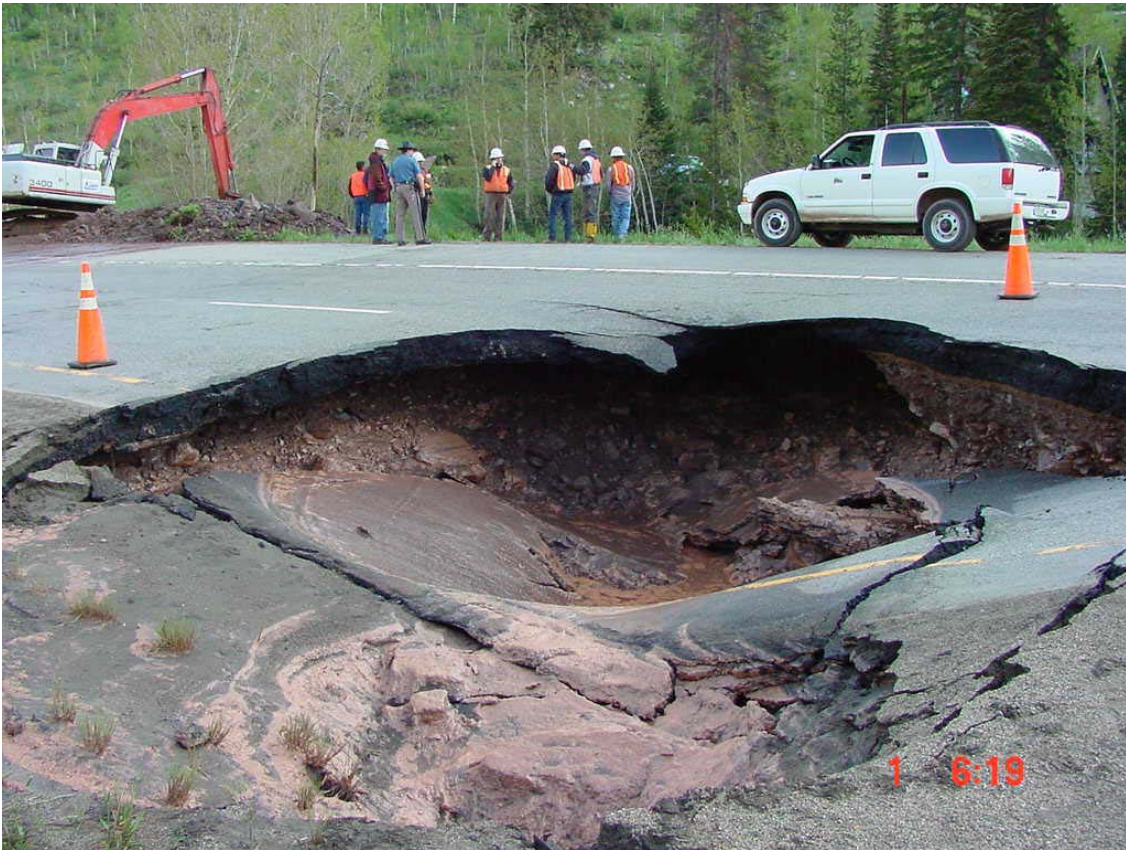
Figure 1.24 –Picture of Interstate 70 Sinkhole Courtesy of Colorado Department of Transportation
