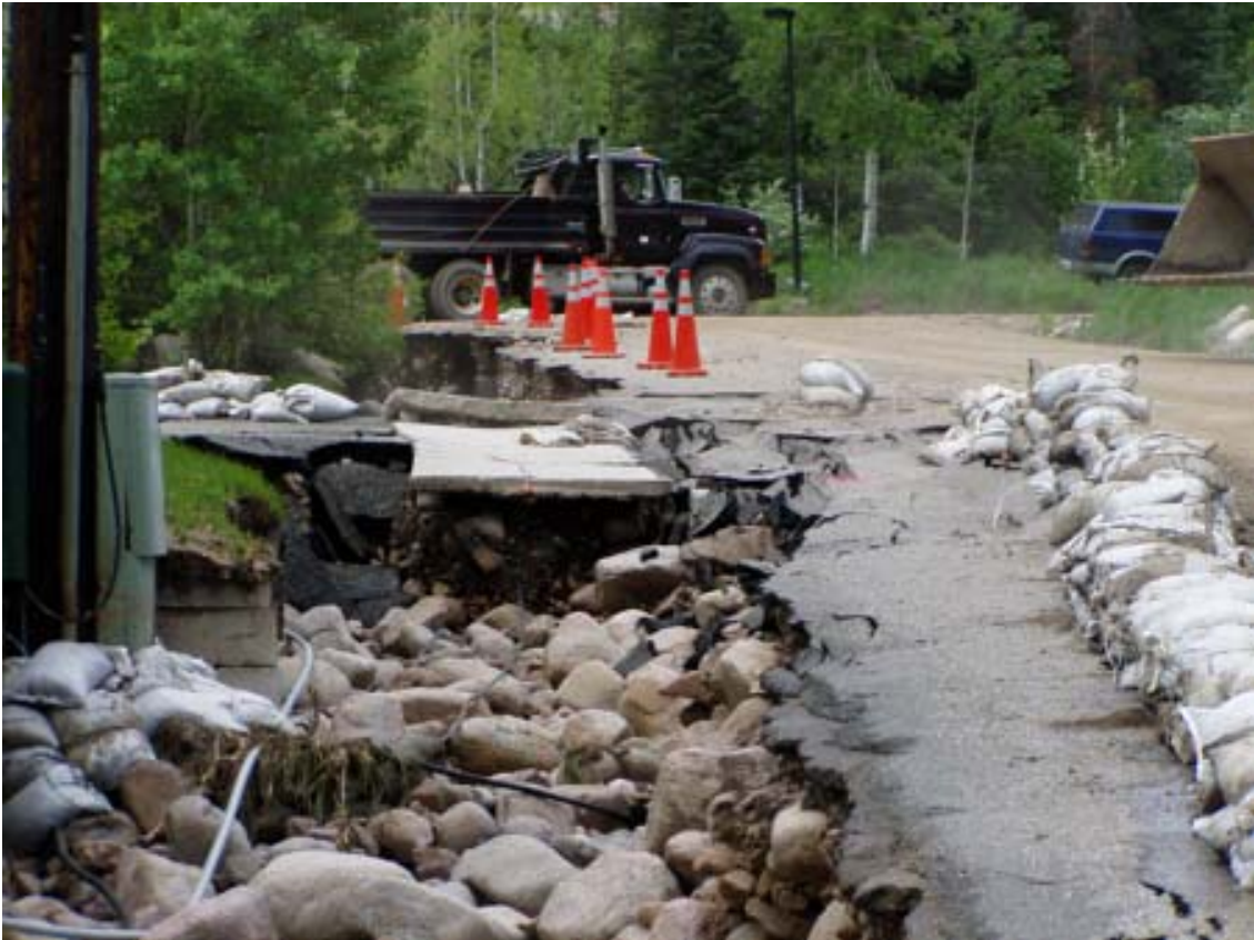
Figure 1.28 –Picture of Damage to Columbine Drive Courtesy of Town of Vail
