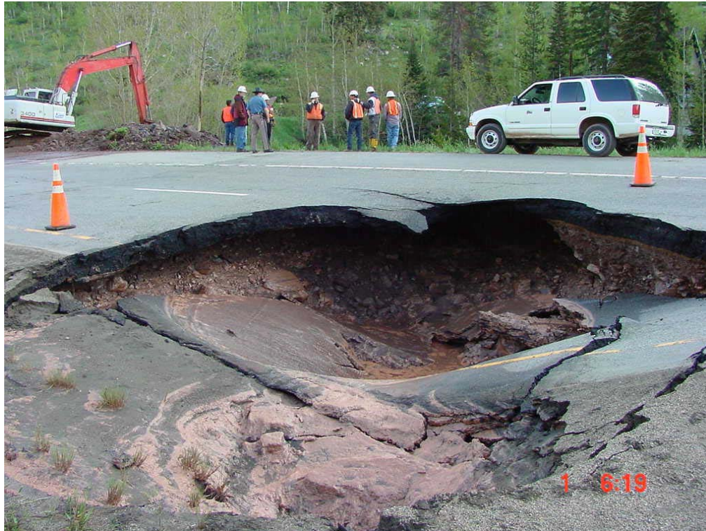
Vail, Colorado Flood of May 31st, 2003 I-70 Drainage Culvert – Bighorn Creek Confluence with Gore Creek Photo Courtesy of Colorado Department of Transportation.
