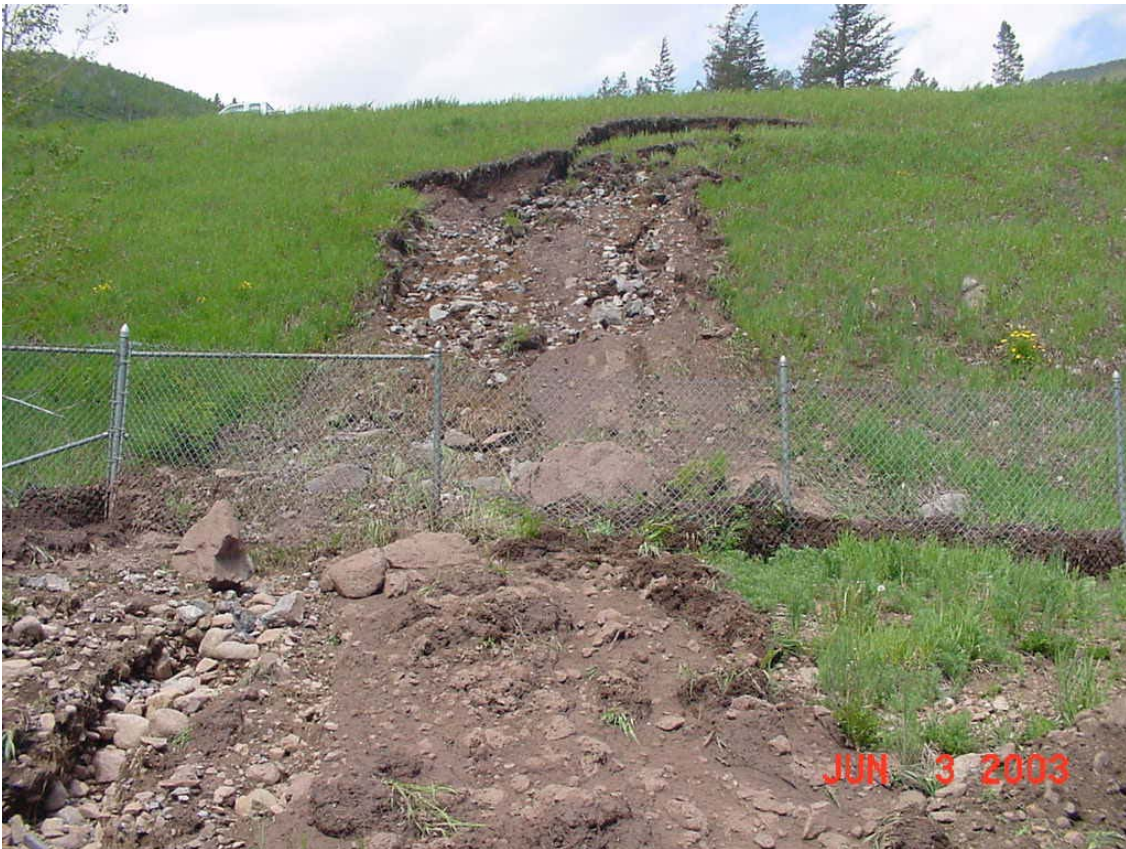
Figure 1.27 –Picture of Hillside Erosion Along I-70 at Mile Marker 181 Courtesy of Colorado Department of Transportation
