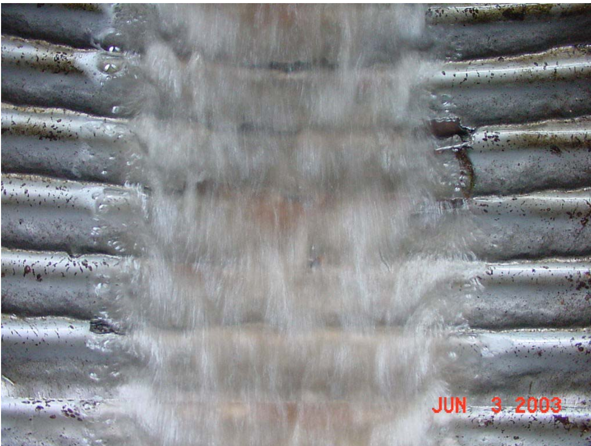
Figure 1.25 –Picture of Corrugated Metal Pipe Degradation at I-70 Culvert Courtesy of Colorado Department of Transportation
