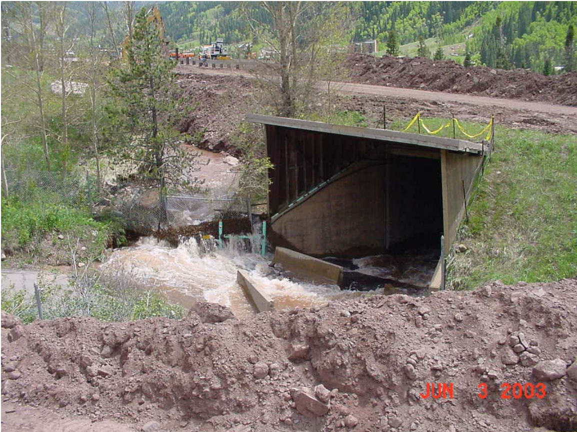
Figure 1.26 –Picture of Culvert at Columbine Drive Underpass Courtesy of Colorado Department of Transportation
