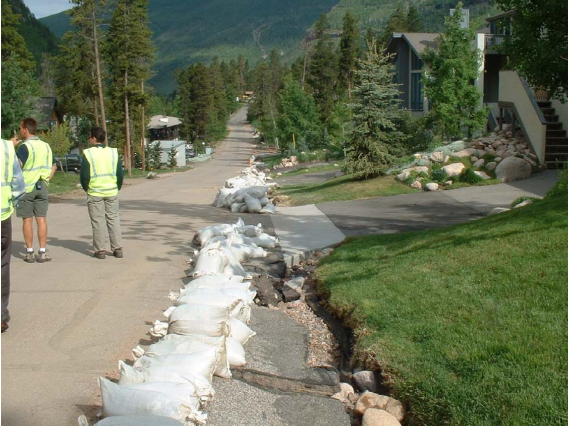
Figure 1.31 – Picture of Erosion Damage to Spruce Way Courtesy of Site Visit by ICON Engineering, Inc.
