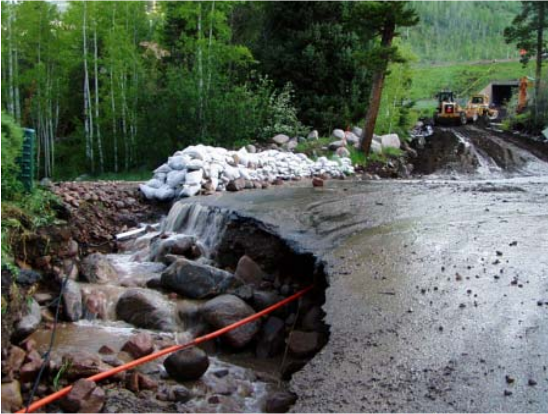
Figure 1.29 –Picture of Damage to Columbine Drive below Interstate 70 Courtesy of Town of Vail
