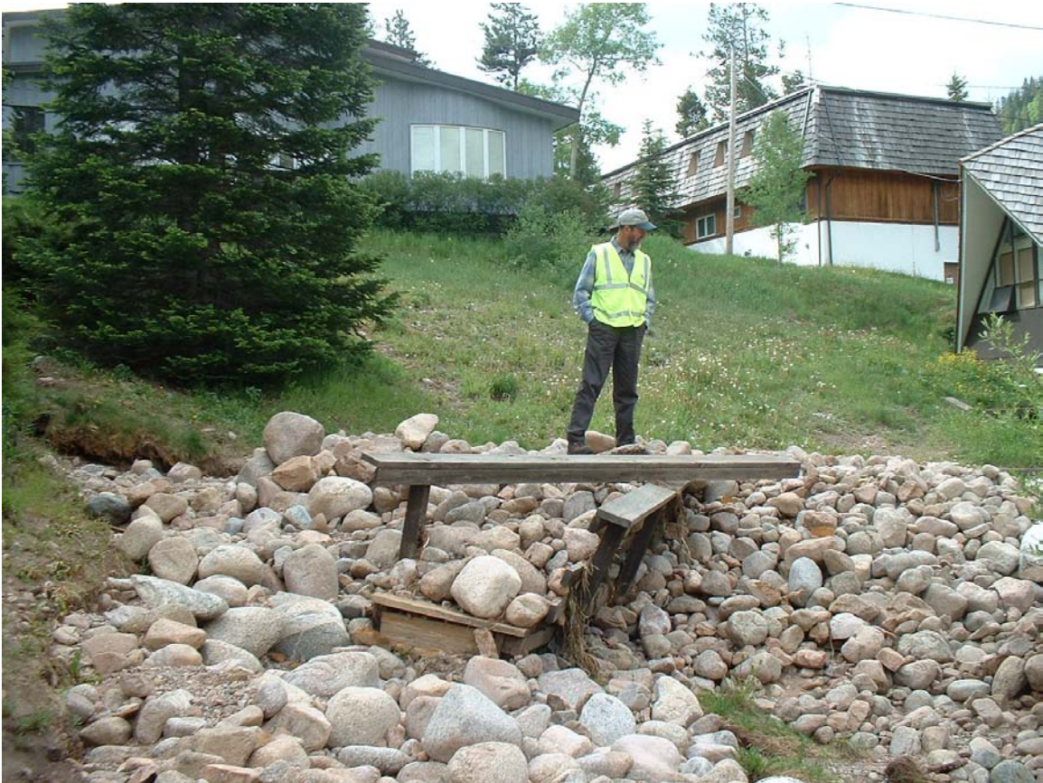
Figure 1.31 –Close-up Picture of Debris Pile at Pond near Columbine Drive Courtesy of Site Visit by ICON Engineering, Inc.
