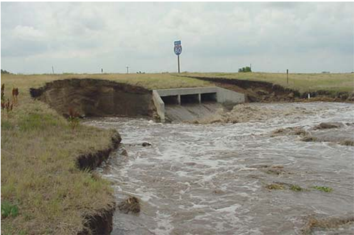
Figure 7.29 – Erosion Damaged Spillway Along Interstate 80. Picture courtesy of the Nebraska DOT.
