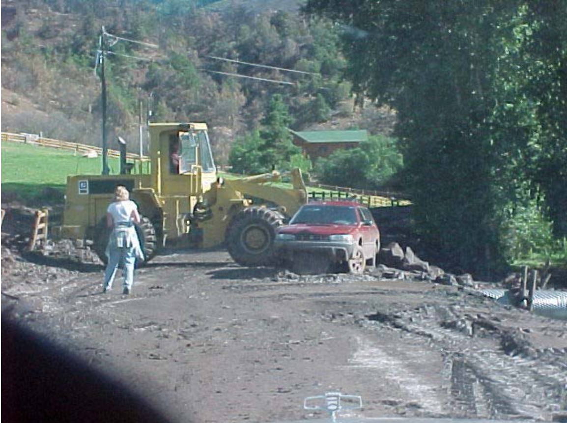
Figure 5.22 – Picture of Mitchell Creek Road During Cleanup Efforts After the Event.
