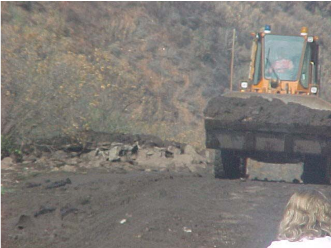
Figure 5.24 – Picture #3 of Mitchell Creek Road During Cleanup Efforts After the Event.
