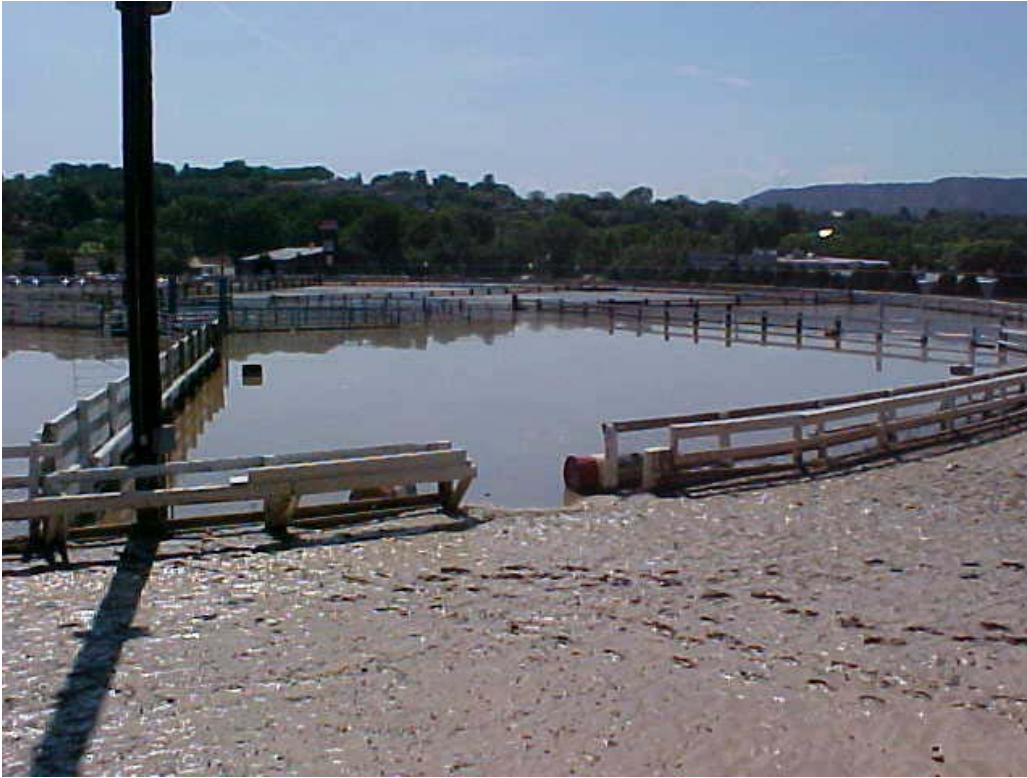
Figure 2.17 – Rifle Fairgrounds Damage Picture 7.
