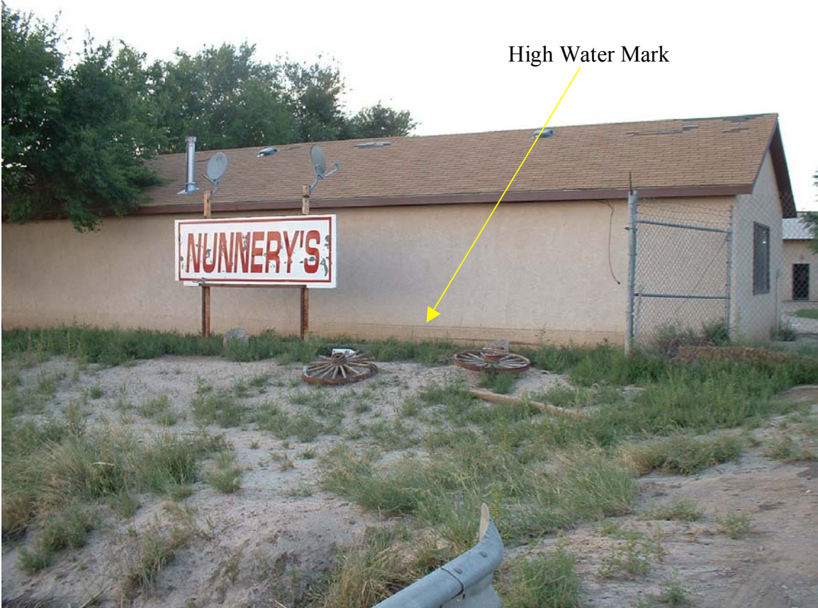
Figure 6.28 – Looking South along Highway 50, in Lamar, at High-Water Line on Structure.
