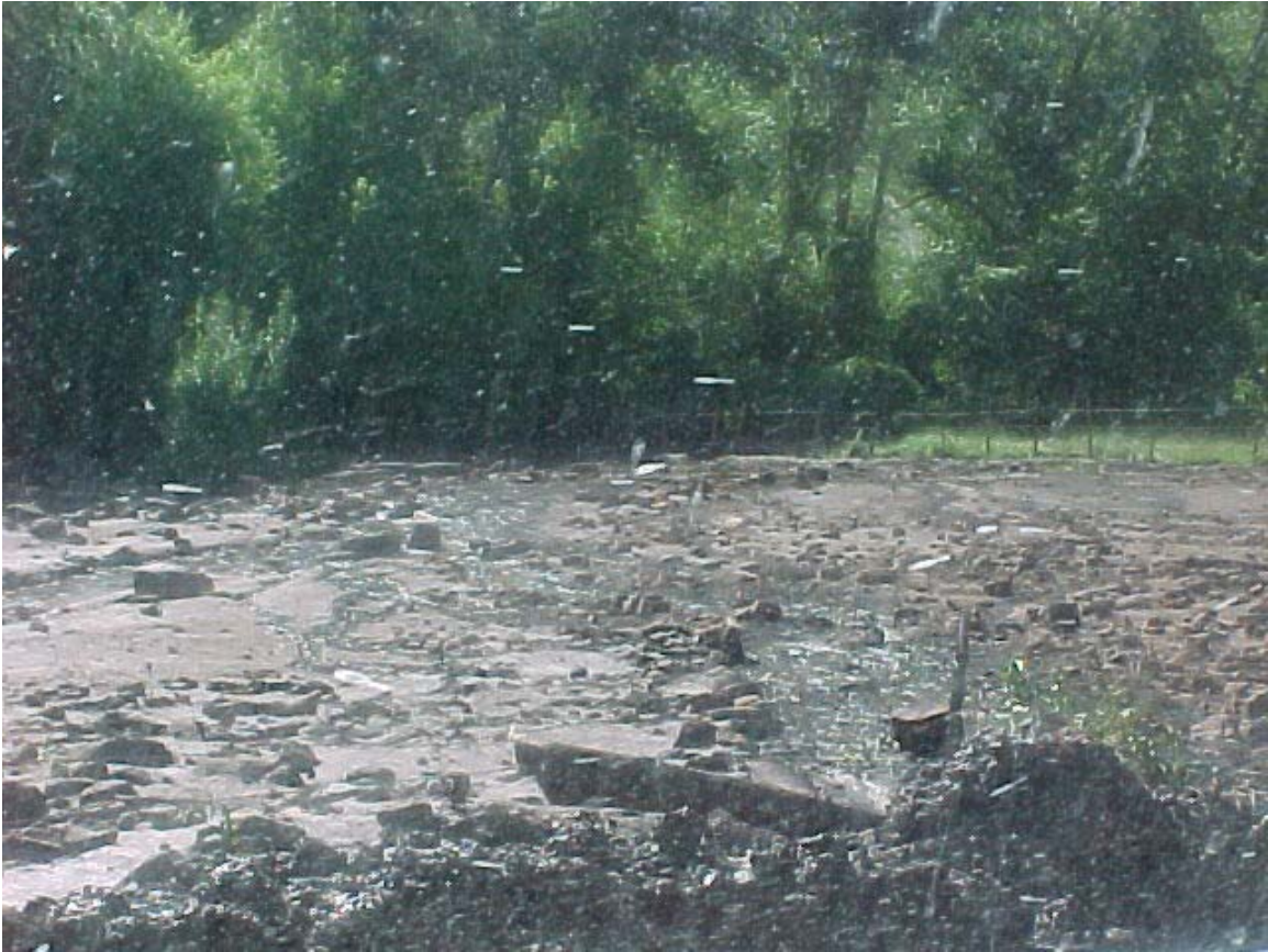
Figure 5.25 – Picture #4 of Mitchell Creek Road During Cleanup Efforts After the Event.
