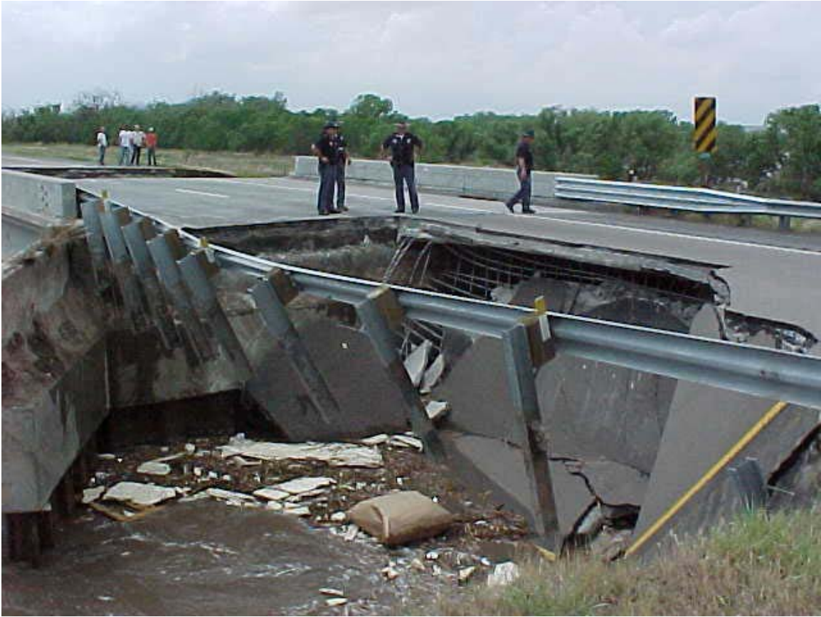
Figure 7.24 – Close-Up Picture of Flood Damage to Bridge on I-80. Picture courtesy of the Nebraska DOT.
