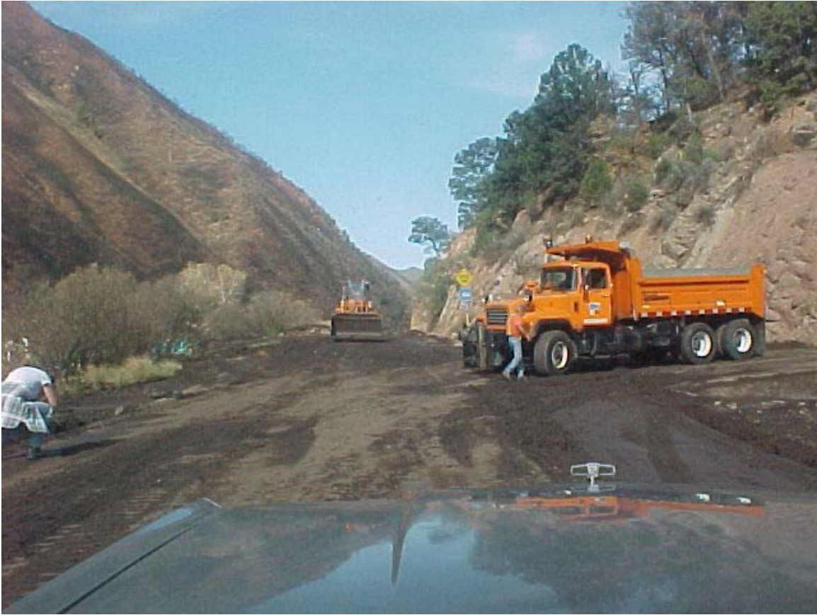
Figure 5.23 – Picture #2 of Mitchell Creek Road During Cleanup Efforts After the Event.
