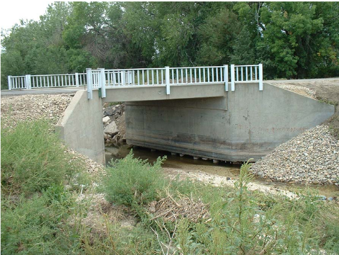
Figure 6.22 – Highway 196 Bridge in Wiley, Colorado Looking South After the Flood.
