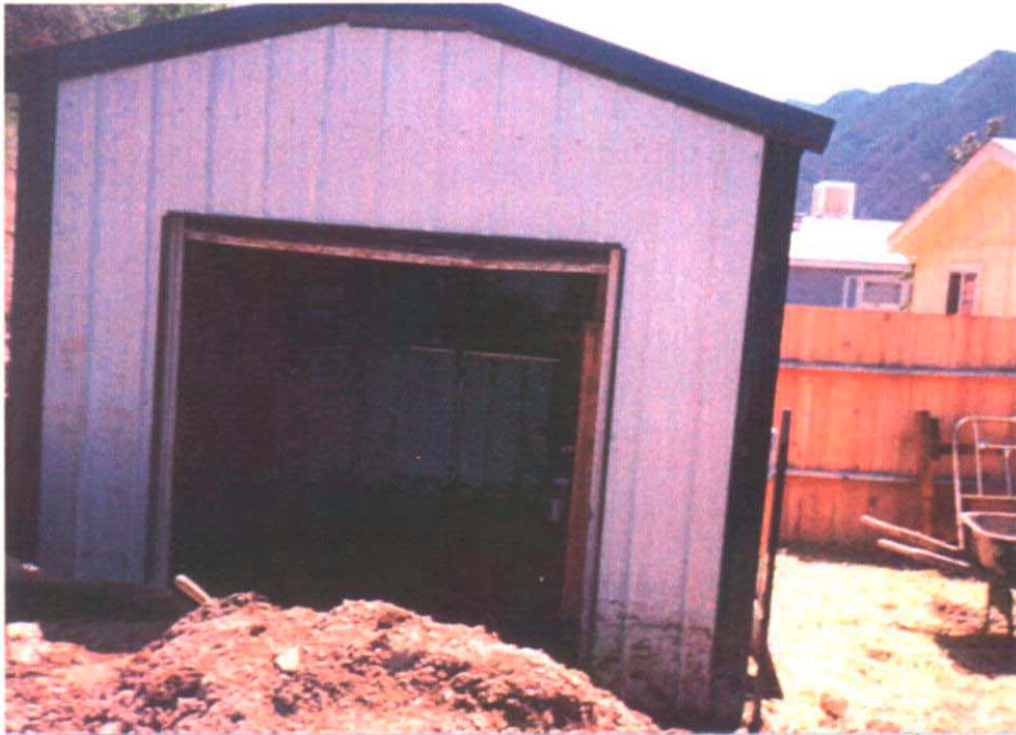
Further examples of residential flood damage in the City of New Castle
