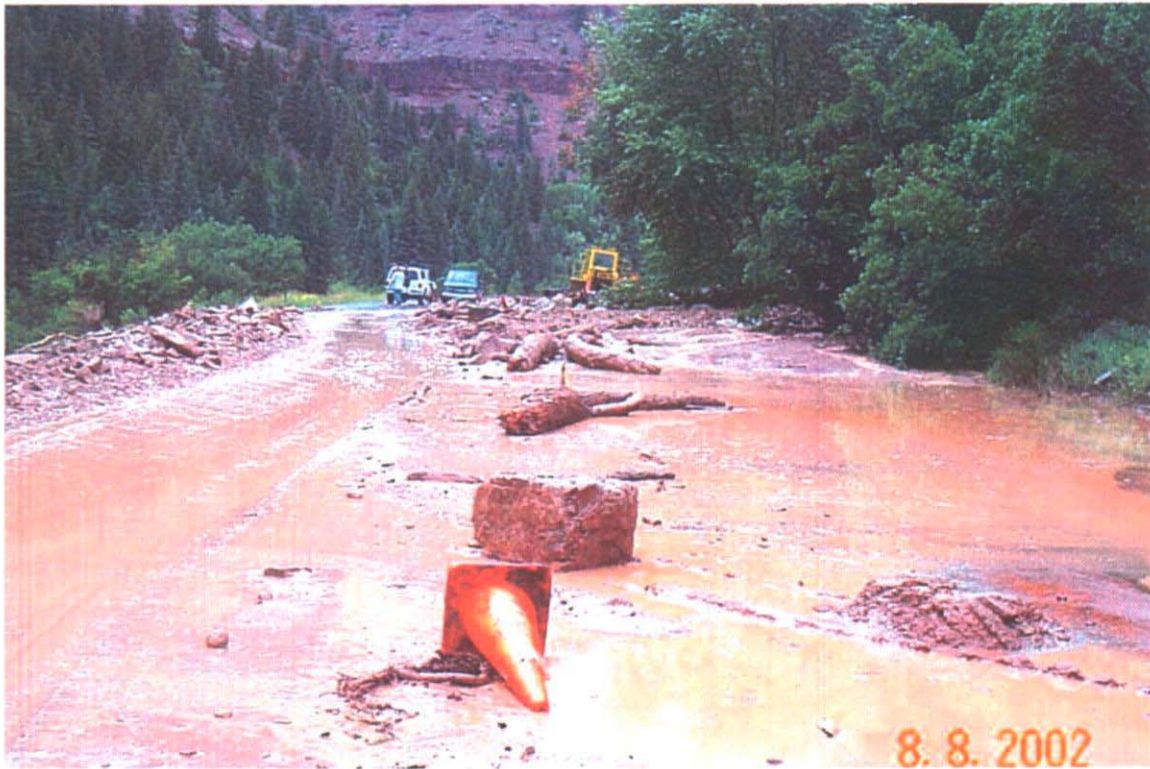
Types of drainage and the resulting overflow along State Route 145 near the City of Telluride
