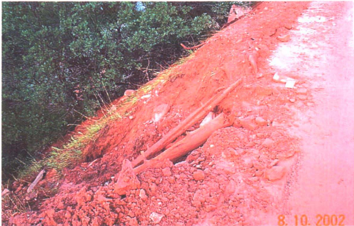
Drainage and embankment deterioration along State Route 145 near Telluride
