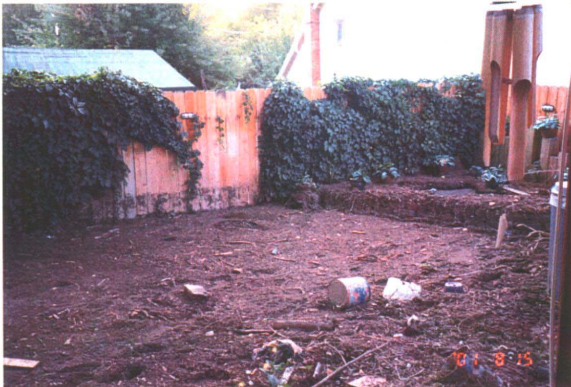
Further examples of residential flood damage in the City of New Castle
