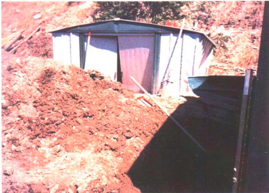
Further examples of residential flood damage in the City of New Castle
