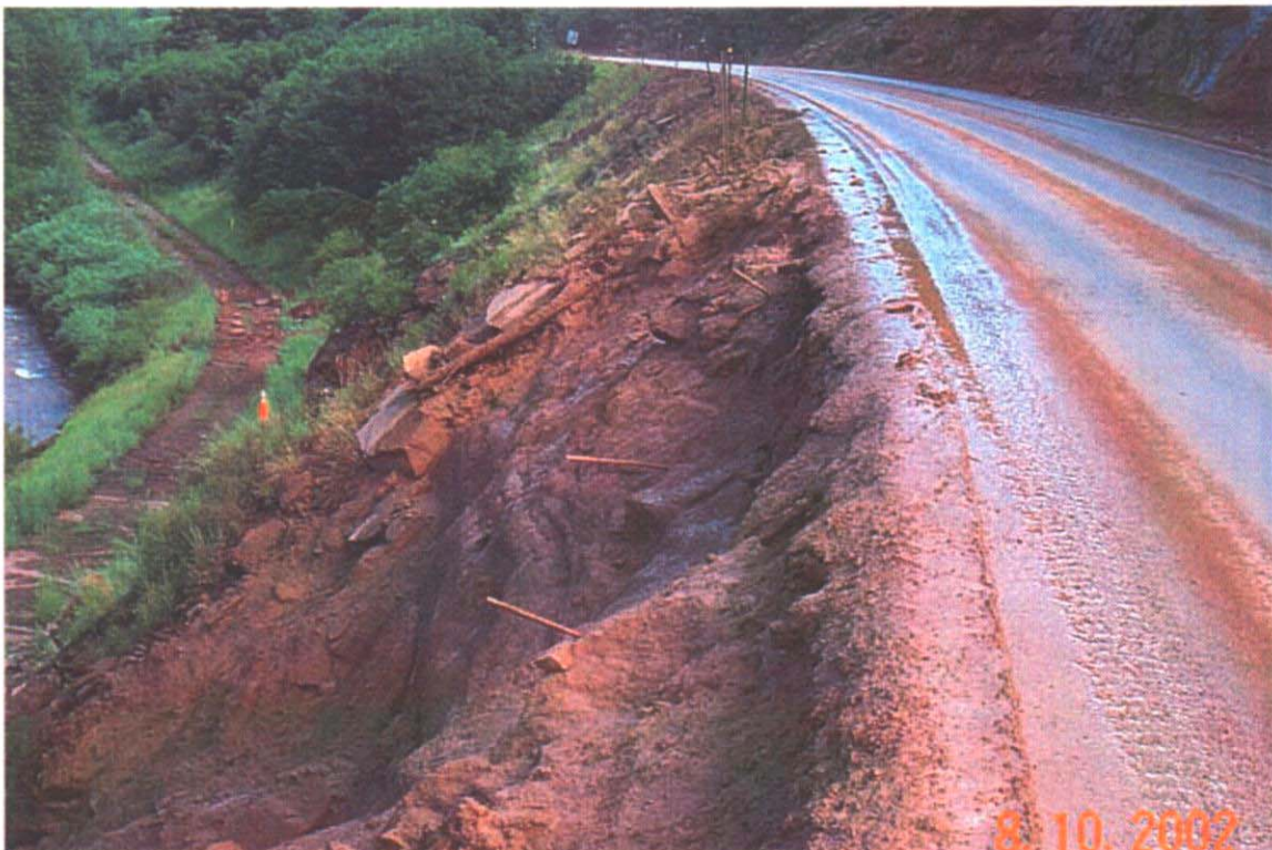
Embankment deterioration along State Route 145 near Telluride
