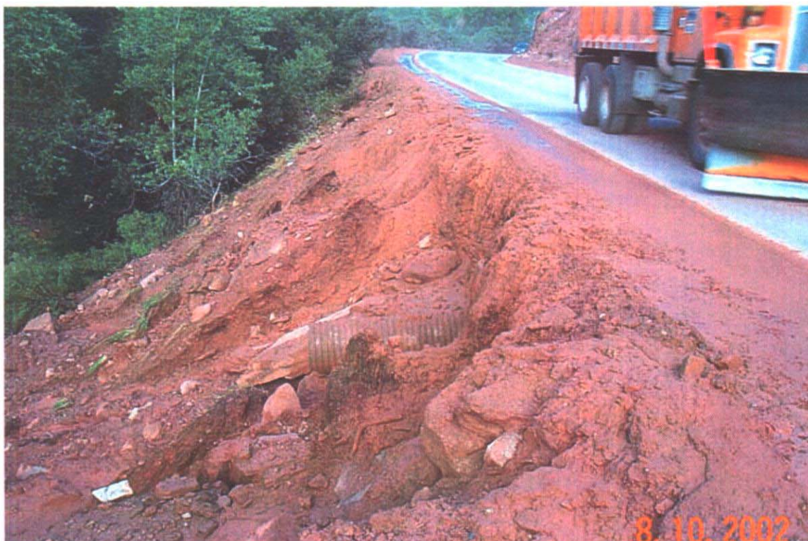
Drainage and embankment deterioration along State Route 145 near Telluride
