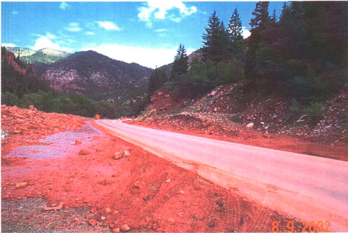
Drainage and the resulting overflow along State Route 145 – Telluride vicinity
