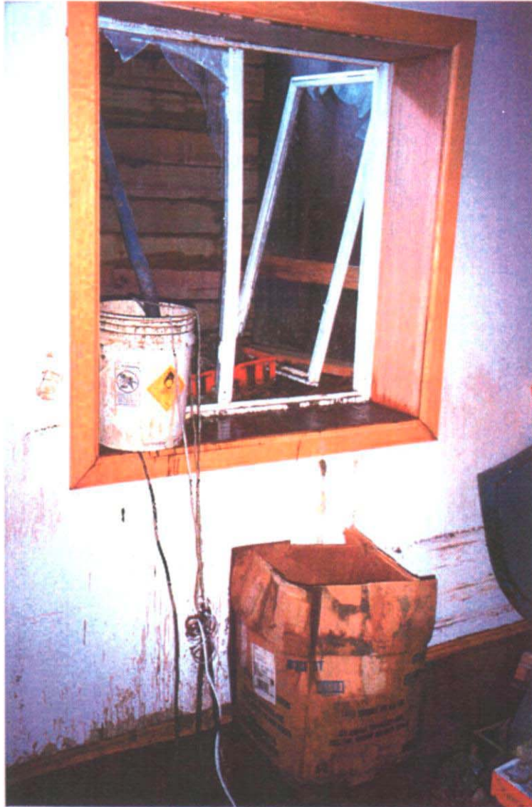
Further examples of residential flood damage in the City of New Castle
