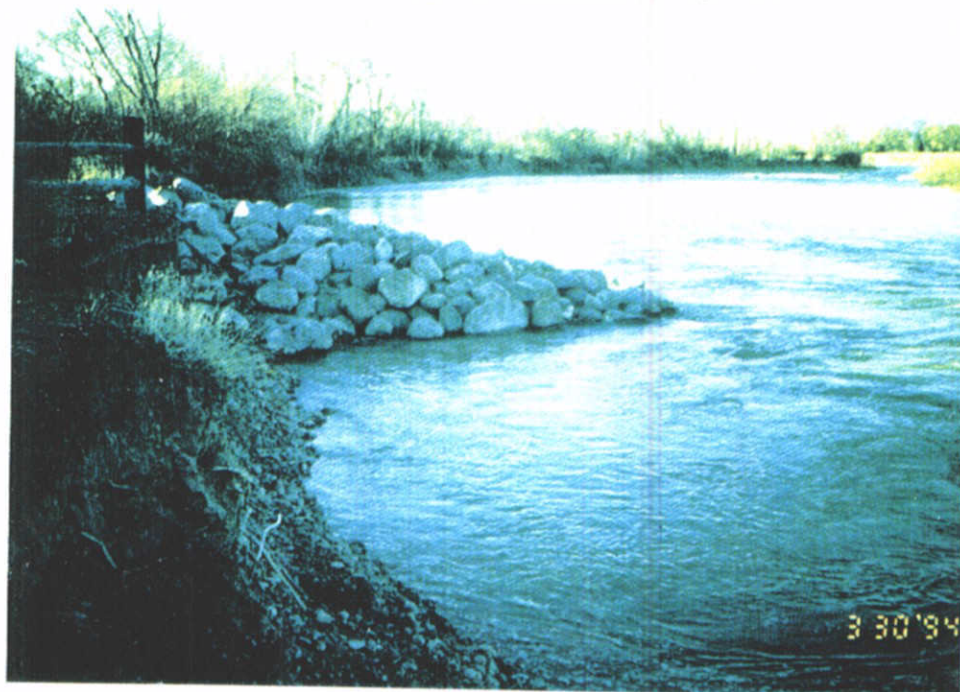
Photo No. 4 Rock jetties at the Rosevale Area on the Colorado River completed May 3, 1994
