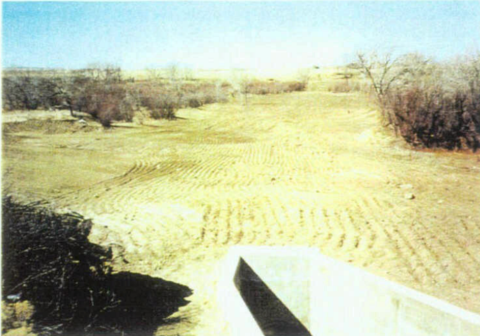
The Concrete Siphon Outlet Structure Looking West Across the Purgatoire River Valley
