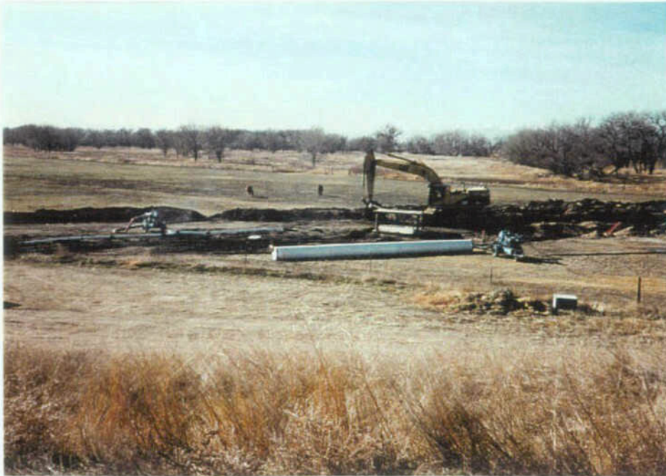
Laying the 28" Steel Pipe from West to East, Just East of the S. Platte River Near Platteville
