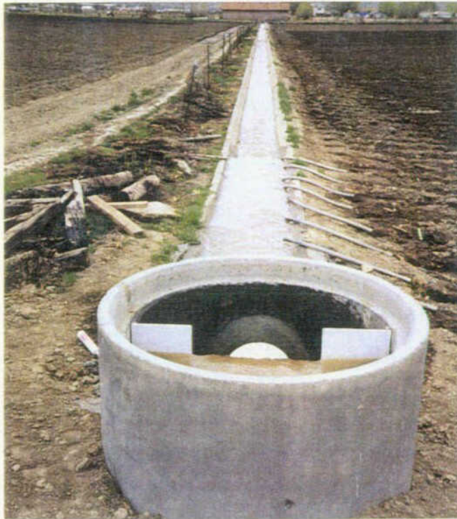
Typical 48" Standpipe Field Turnout along the Appleton Ditch
