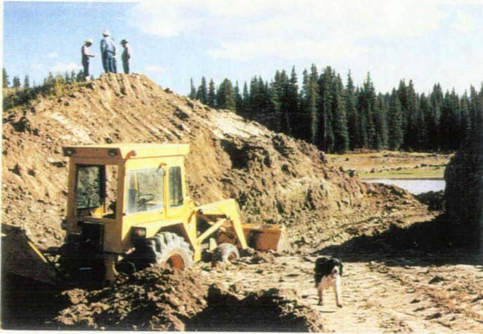
Military Park Reservoir Breached Dam
