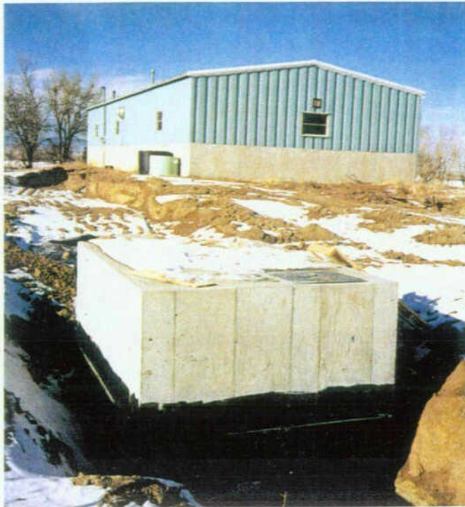
Raw Water Inlet Control Vault at the Erie Water Treatment Plant
