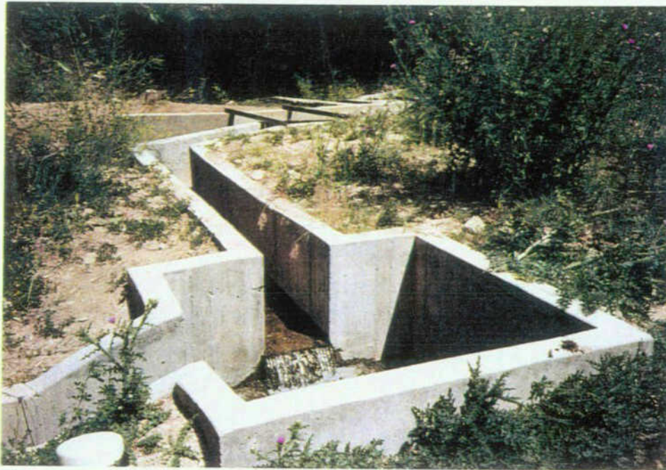
Kingsrow Homeowner's Diversion Structure/Division Box
