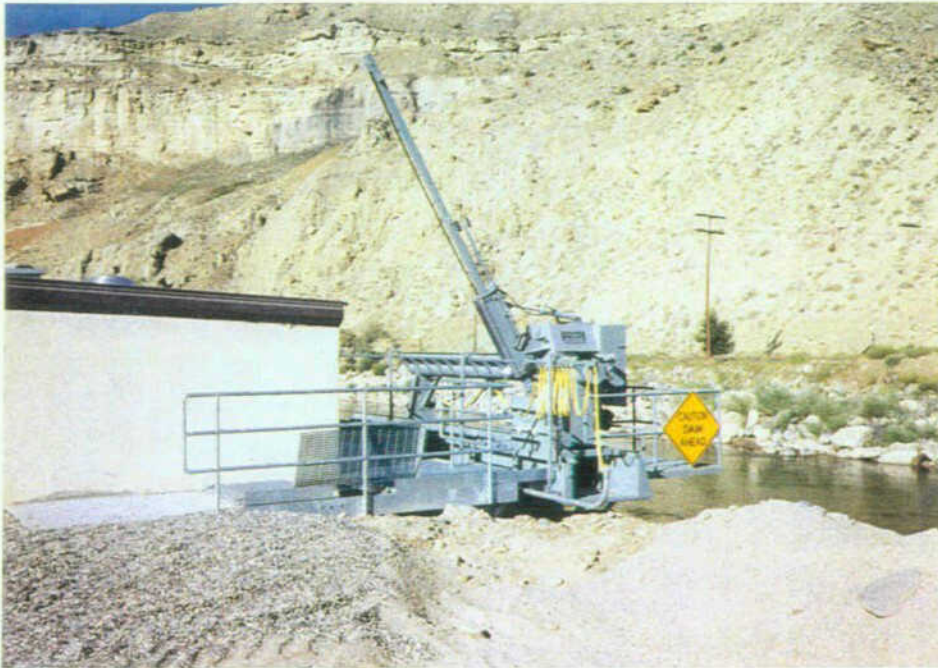
Automatic Trash Rack at Pump Station Intake
