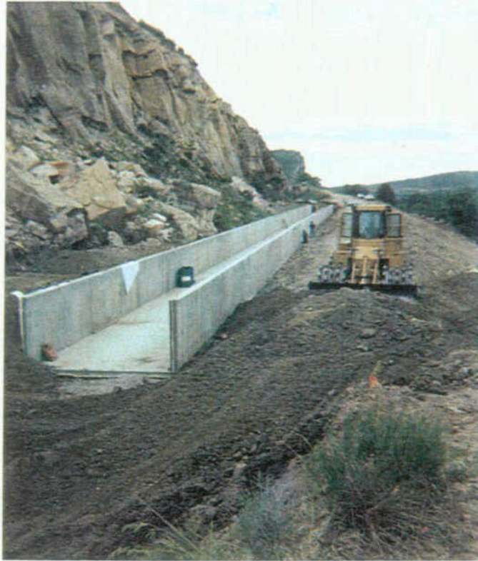
The Poudre Valley Canal Under Construction looking south just east of U.S.287
