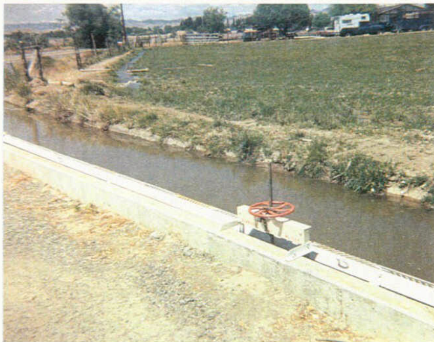
Elmwood Lateral Ditch Headgate
