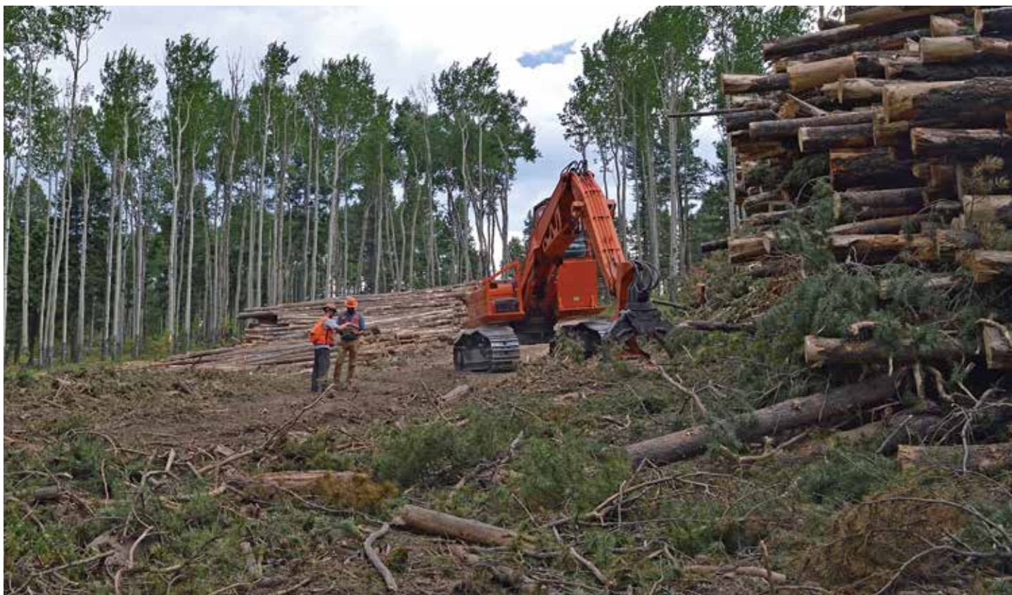
CSFS foresters Max Erickson and John White assess wood harvested during the Heavens Project. The CSFS engaged the wood products industry to ensure trees felled during the project became saw logs, firewood and wood chips for a biomass power plant. Photo: Nathan Beckman, CSFS
