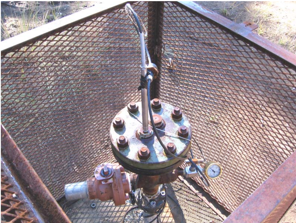
Monitoring Well MW 35-6-17-2 Wellhead with External 1000 PSIA Pressure Transducer
