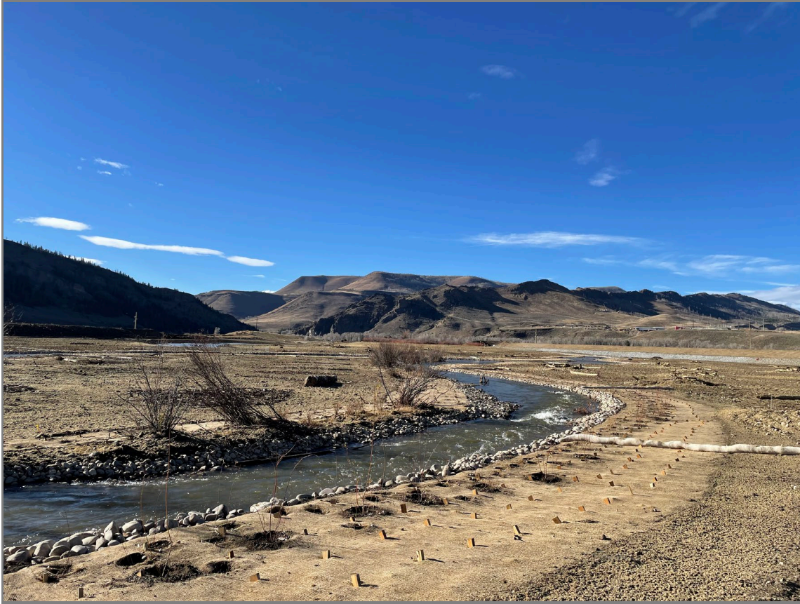
Figure 6. The Colorado Connectivity Channel looking downstream through the former bed of Windy Gap Reservoir.
