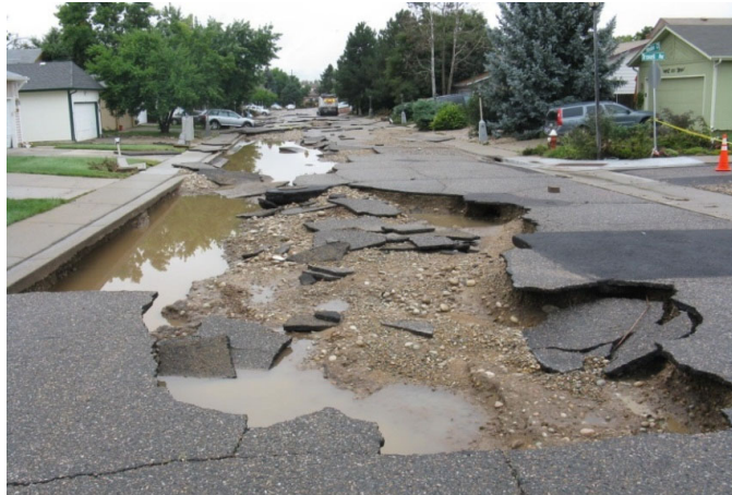
Figure 7: Damage to Hayden Court, Longmont (Source: Survey)
