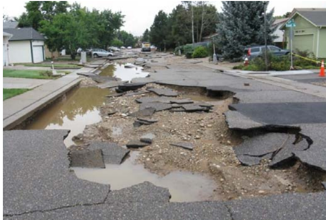
Figure 7: Damage to Hayden Court, Longmont (Source: Survey)
