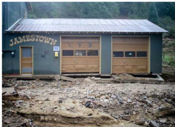
Figure 8: Volunteer fire department in Jamestown damaged from flooding.
