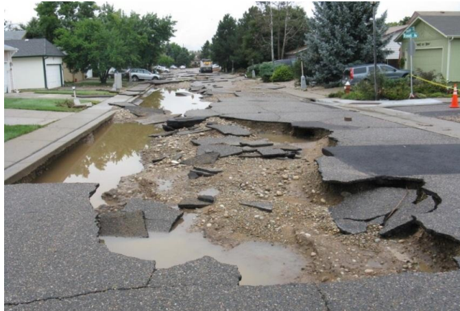
Figure 7: Damage to Hayden Court, Longmont (Source: Survey)
