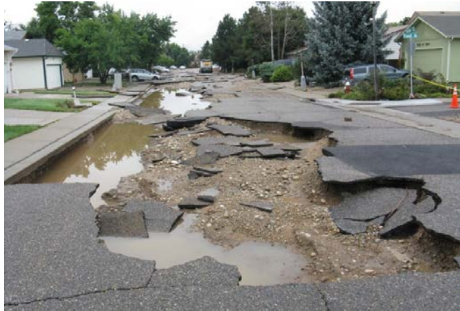
Figure 7: Damage to Hayden Court, Longmont (Source: Survey)
