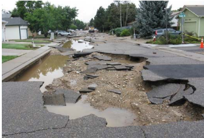
Figure 1: Damage to Hayden Court, Longmont (Source: Survey)
