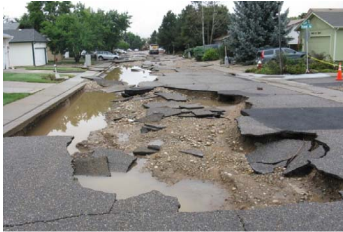
Figure 1: Damage to Hayden Court, Longmont (Source: Survey)
