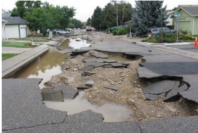
Figure 1: Damage to Hayden Court, Longmont (Source: Survey)
