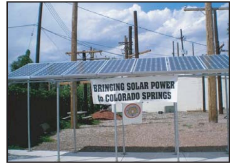
Finished solar panels installed by the apprentices of the Joint Apprenticeship Training Committee
