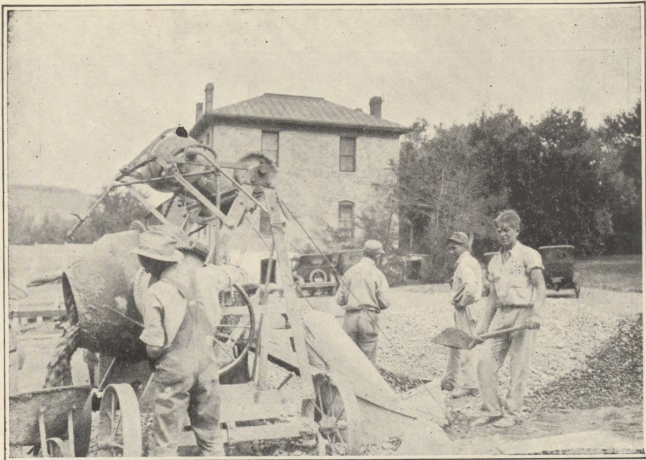
A group of Boys turning out Concrete Work for the New Boiler House
