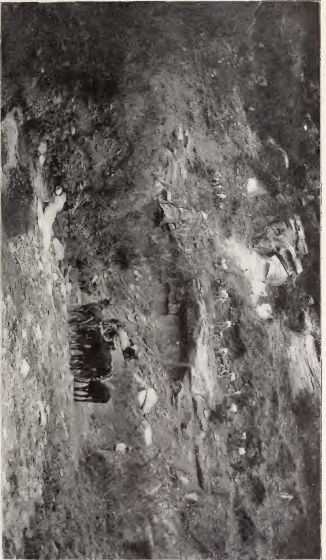
ANOTHER VIEW OF THE "ROAD" BEFORE WORK WAS COMMENCED BY THE CONVICTS FROM THE PENITENTIARY.
