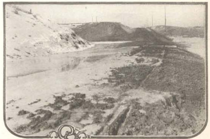
Ice blocks solid the culvert's mouth.
