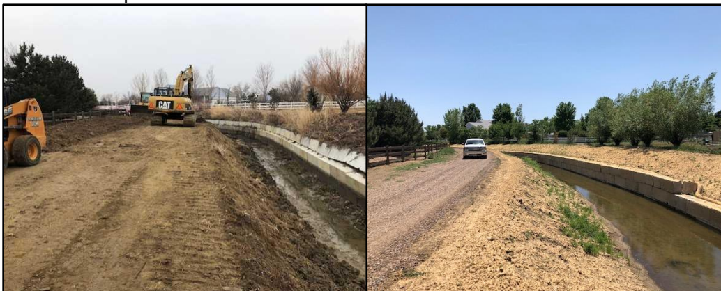
Figure 3. Retaining Wall Between W. 72 nd Ave. and W. 74 th Ave. East of Quaker St. Before (left) and After (right) Repairs
