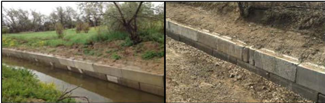
Repair of Block Wall Near 74 th and Quaker. Before (Left), and After (Right).
