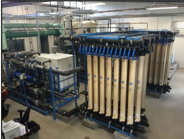
New Microfiltration System at Dory Hill Plant
