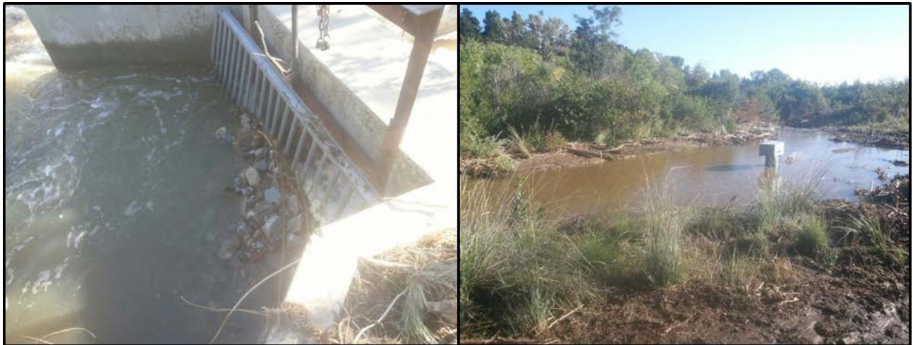
Examples of Flood Damage to KDPL. Headgate Blocked by Rocks and Debris (Left). The Flume is Silted in and the Recorder is Stranded (Right)
