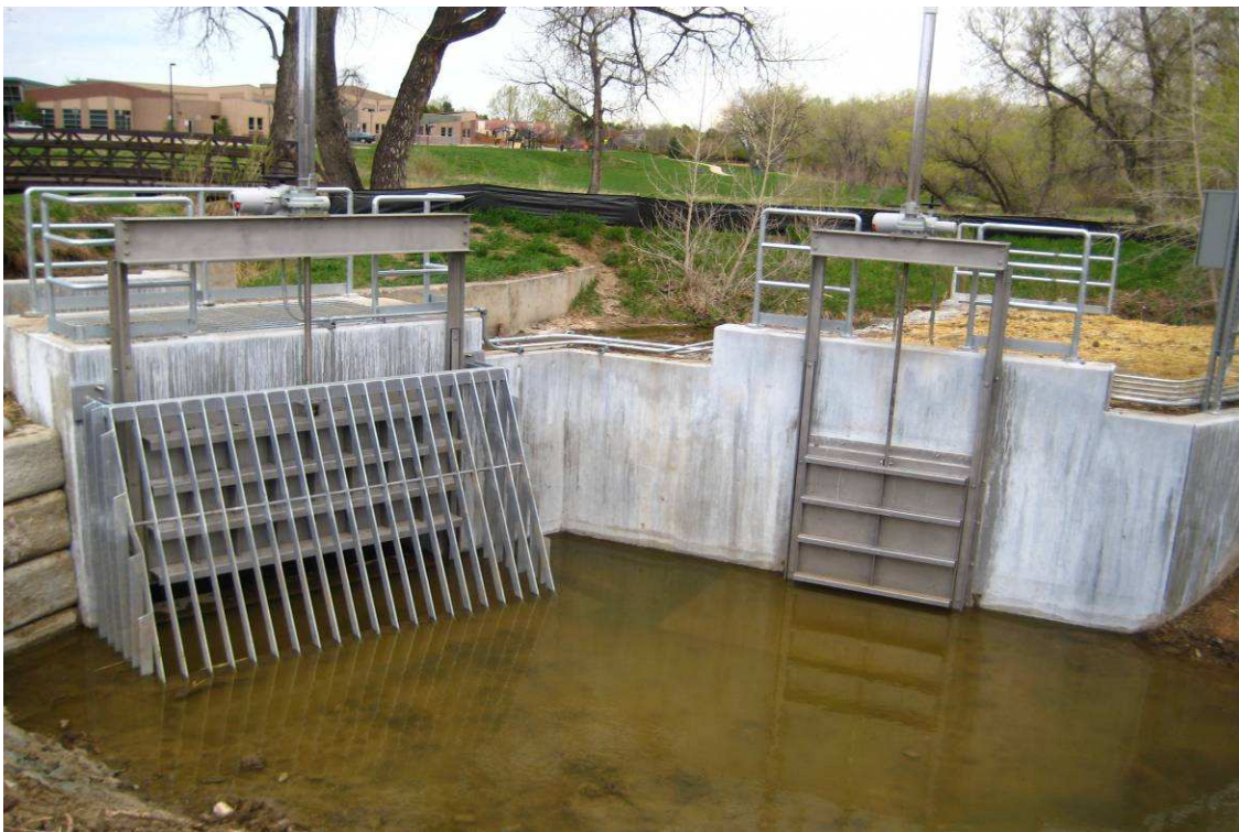
Figure 27. New Church Ditch separator at Little Dry Creek. Ditch is diverted under Little Dry Creek through the structure on the left. The sandout gate on the right returns water to Little Dry Creek in the background.
