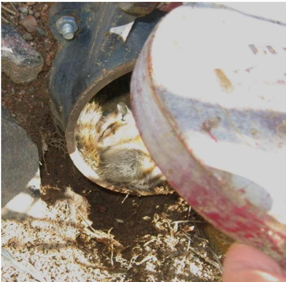
Chipmunk nested in overflow pipe.
