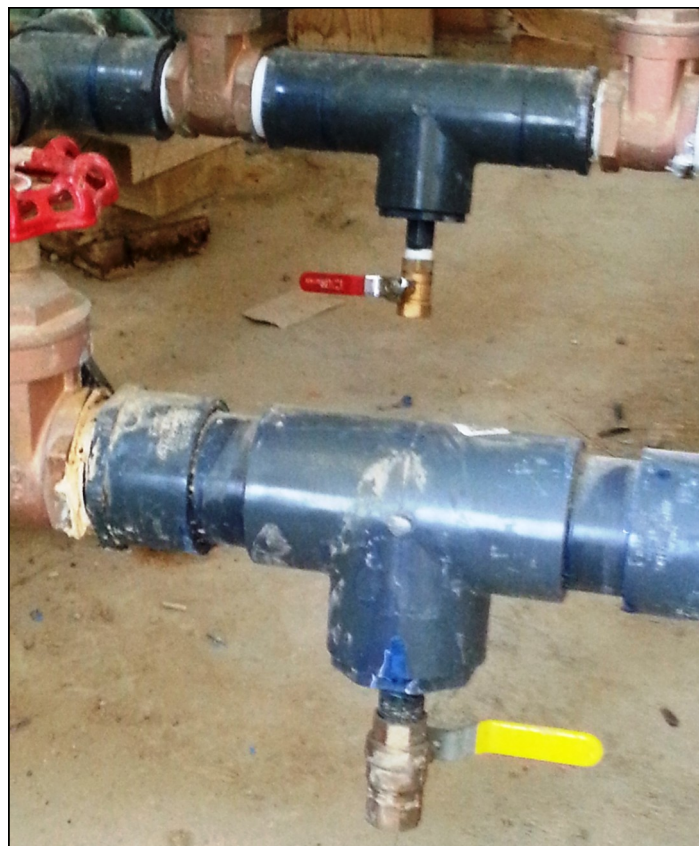
Raw water taps for two wells.
