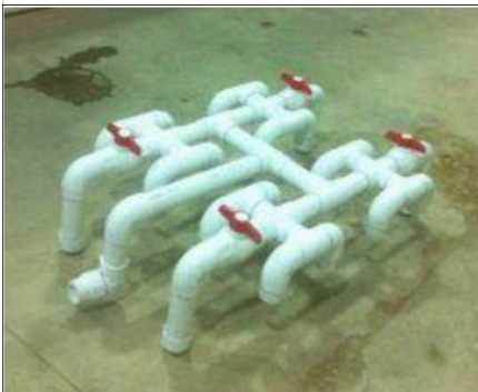
Sixteen inlet manifold
