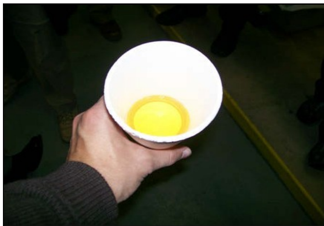
Propylene glycol, the presumed contaminant, drawn from a spigot in the Printers Park Medical Plaza mechanical room.
