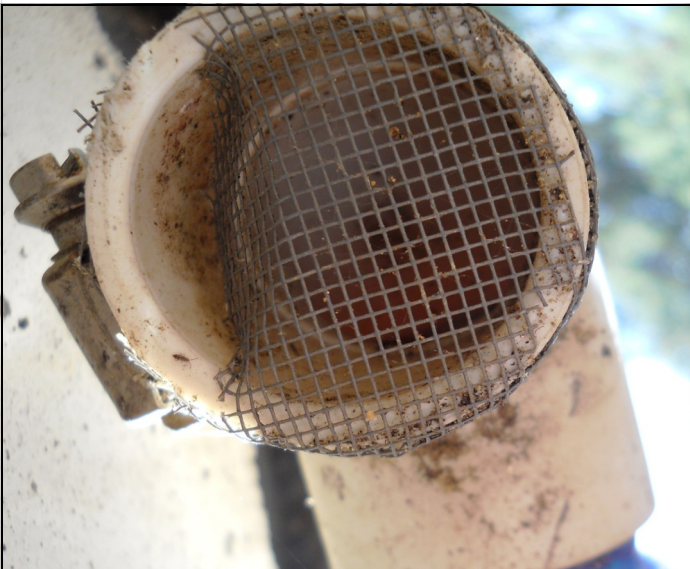
Improperly screened vent
