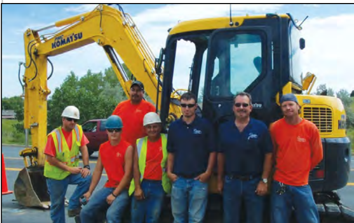
Consolidated Mutual stops to pose for a picture while installing an 8-inch mainline
