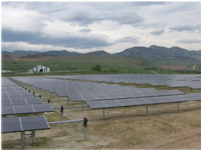
Photos of Ralston Water Treatment Facility solar field
