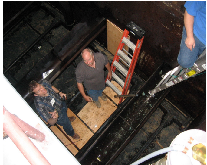
Filter surveillance is an important part of operating and maintaining a conventional or direct surface water treatment process. Students in the advanced training sessions learn to apply these skills in a filter basin like this one at Ute Water.
