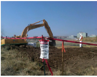
A photo of the remediation of asbestos contaminated soil at the Denver Federal Center
