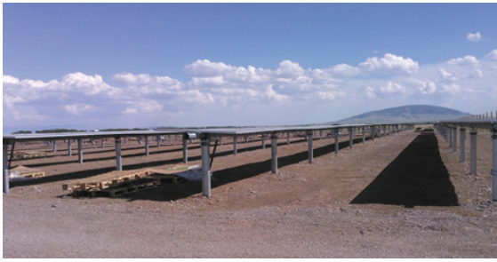
One of two San Luis Valley community solar gardens that offsets energy use at the Summitville Mine.
