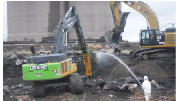
Breaking and removing concrete in former coke batteries at the EVRAZ steel fabricator in Pueblo.
