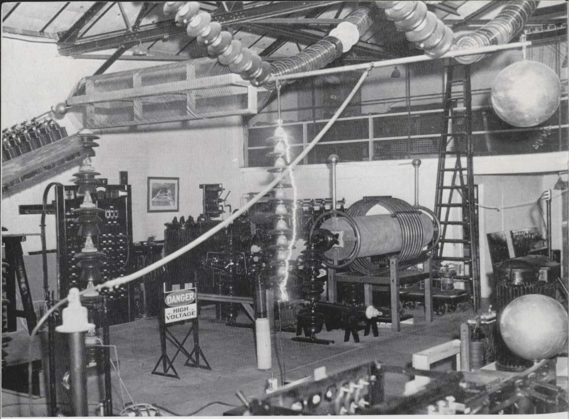
Testing power line insulation with the million-volt lightning generator.
