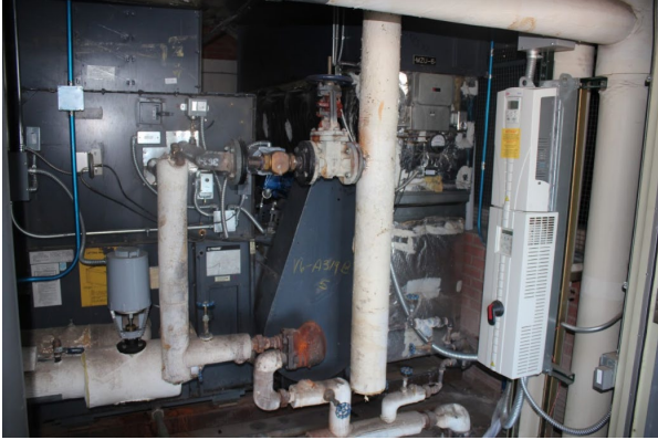
Current HVAC in Bldg. 121
