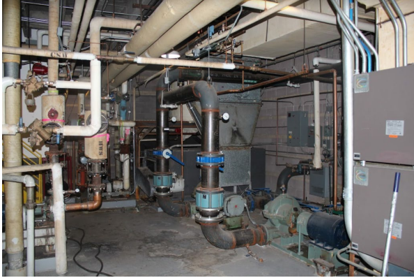
Current HVAC in Bldg. 125
