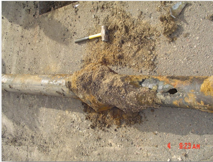
Typical water line corrosion. This line had a hole on the top. Note how the corrosion held to the pipe when removed.
