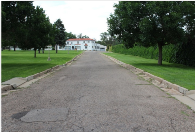
Broken curbs do not provide adequate drainage. Asphalt in poor condition.
