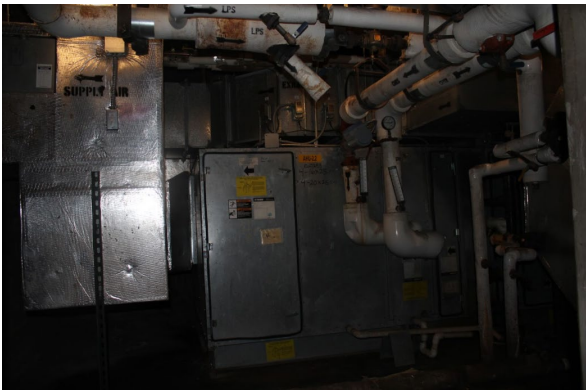
Current HVAC in Bldg. 116
