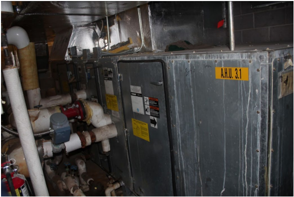
Current HVAC in Bldg. 115
