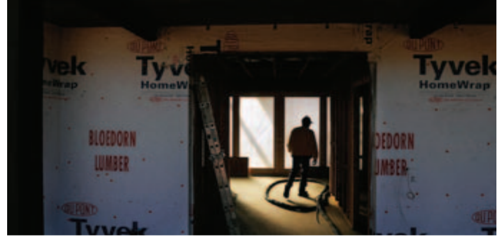
Jim Tanner of B&W Glass of Cheyenne, Wyoming gets supplies as he works to install large skylights in an Energy Star home north of Fort Collins, Colorado being built by L.R. Barker Builders, Inc.
