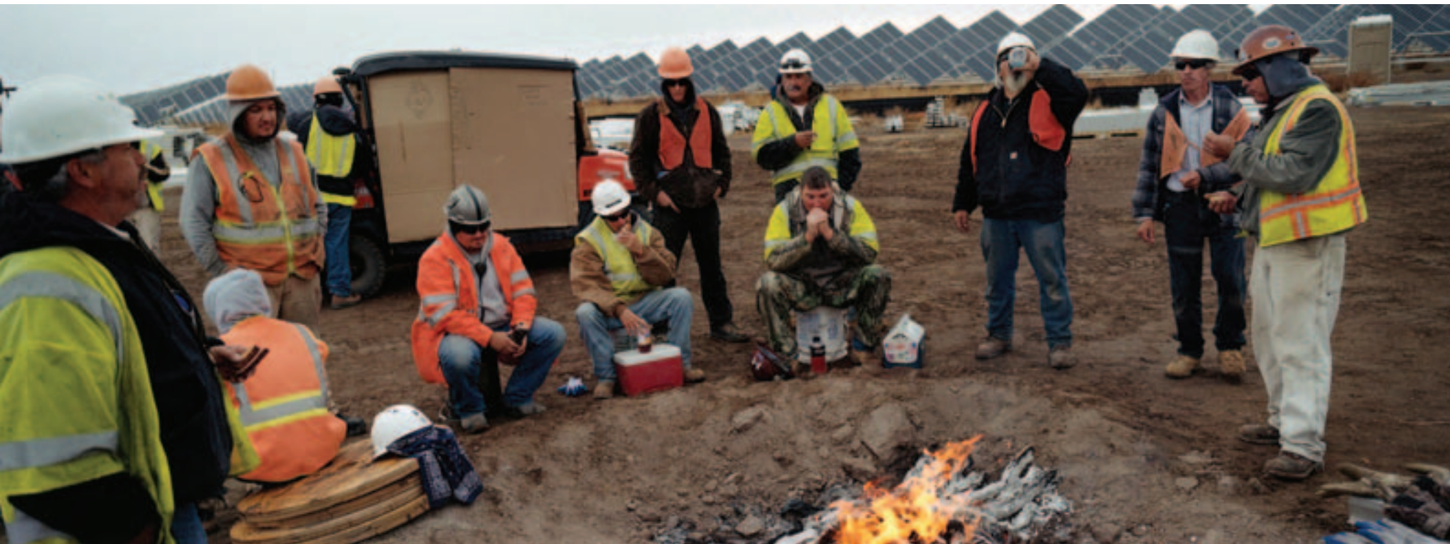
Workers keep warm near a fire during a break while working at the Greater Sandhill Solar Project being constructed by SunPower Corporation outside of Alamosa.
