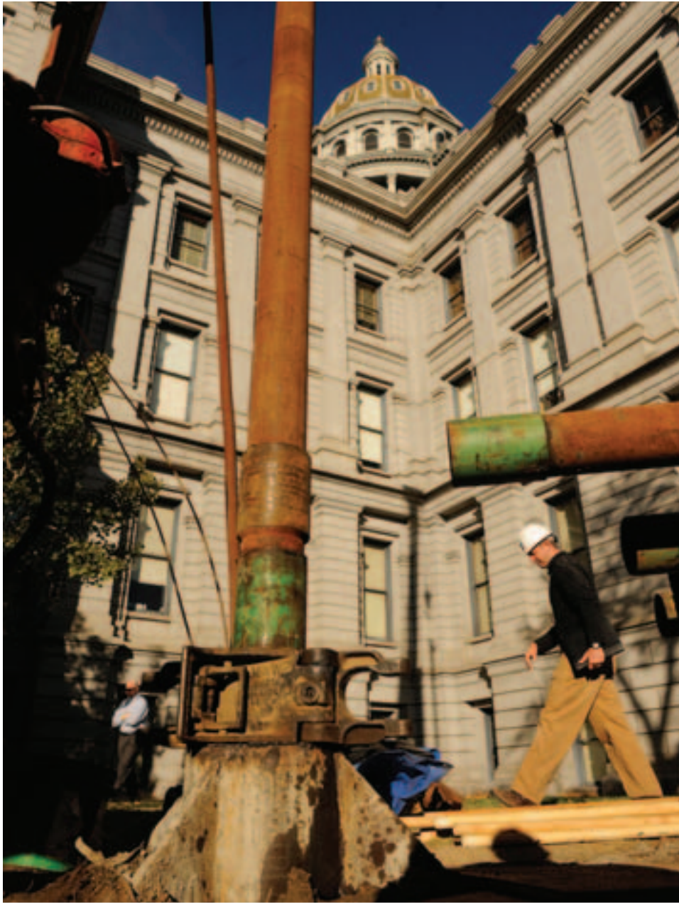
A drill rig is set up for a geothermal project in front of the state capitol in downtown Denver.
