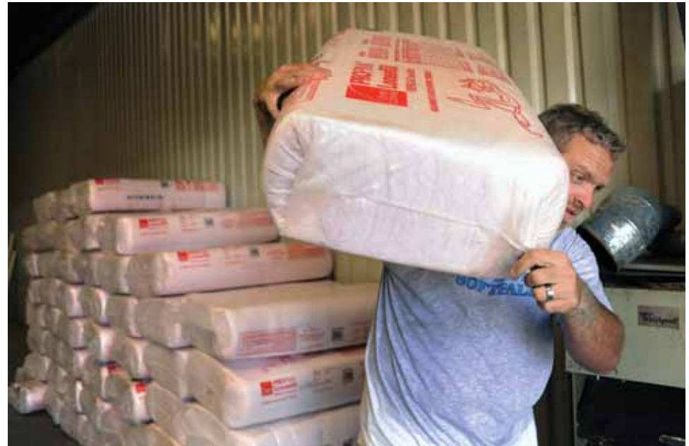
Hank Myers of the Northeastern Colorado Association of Local Governments carries a bag of insulation at a Greeley warehouse as he and other workers weatherize two homes.
