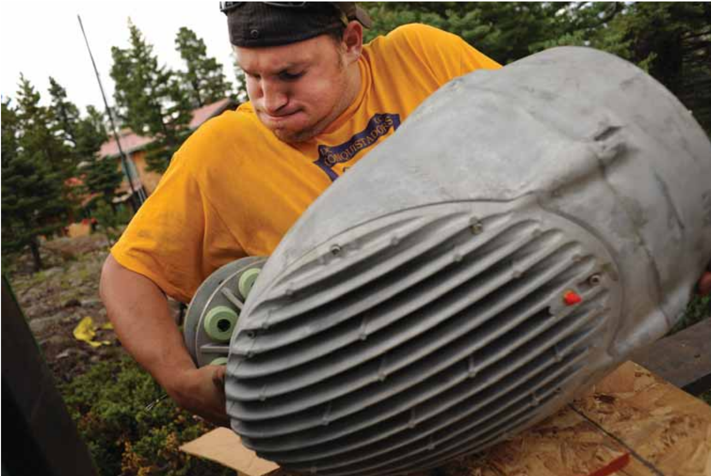
Kyle Remley of Headwaters Energy lifts the head of a windmill assembly during installation at the Westcliffe home of Lou and Betsy Puls.
