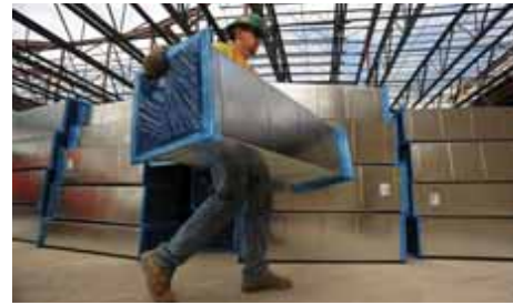
Josh Winegarmer carries a section used for the new, more energy efficient heating and cooling system for Casey Middle School in Boulder.
