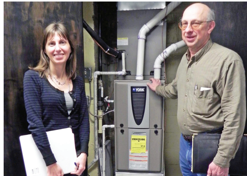
EOC installed a new furnace at a church that provides community outreach services.
